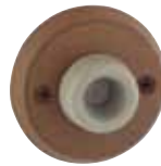
Wrought Steel Wall Bumper Rust
